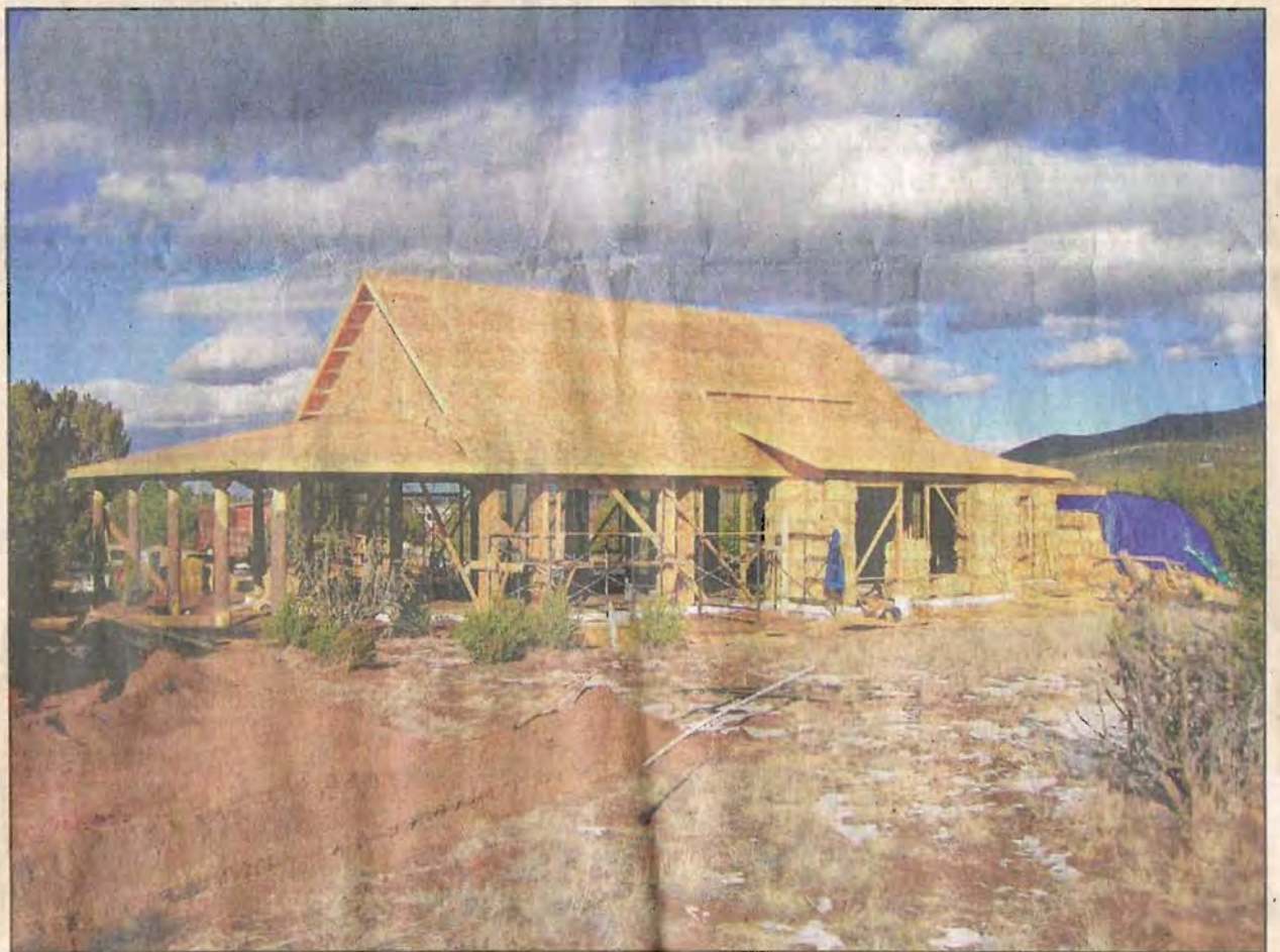
This 1,360-square-foot straw bale home, located at 3 Stagecoach Junction Place in a pre-existing subdivision in the East Mountains, has passive solar glazing and orientation. Wraparound porches and an integrated gray-water system are among the many green features.
